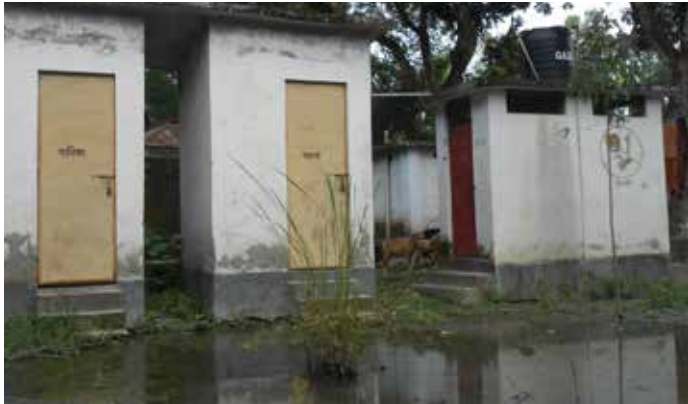
The School Latrine in inundation before social audit
